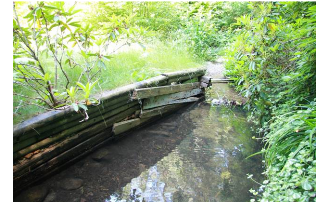
(b) Failing retaining walls on ponds upstream of wood weir dam.
