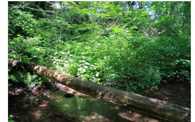
(d) Low-bank area on right bank upstream of LVTC outfall suitable for off-channel pond. Knotweed (seen here in foreground) stands are present throughout this area and require management.
