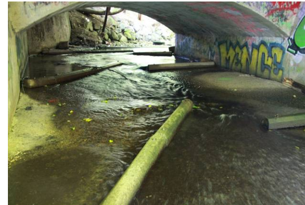
(a) Existing no-post barriers to aid in fish passage under Mountain Highway bridge.
