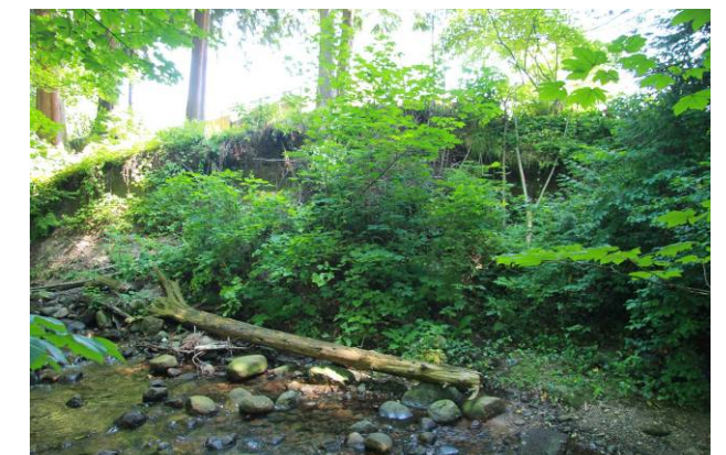
(f) Bank erosion and instability on left bank of Coleman Creek upstream of Harold Rd footbridge.
