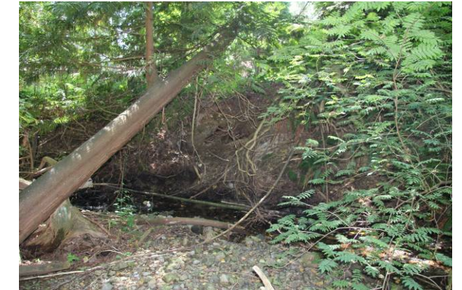
(b) Area of bank erosion on right bank at “bubble pool” opposite Donovan Pond.
