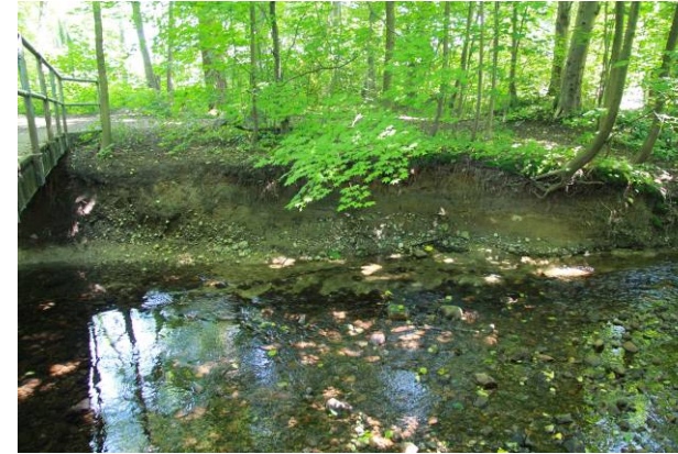
(a) Bank erosion below footbridge at lower Argyle School playing field.
