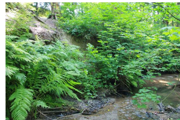
(e) Bank erosion and instability on left bank of Coleman Creek downstream of Harold Rd footbridge.
