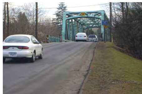
Missing sidewalks at Keith Road Bridge
